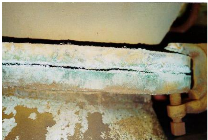
Building 410 corroded ash receiver
