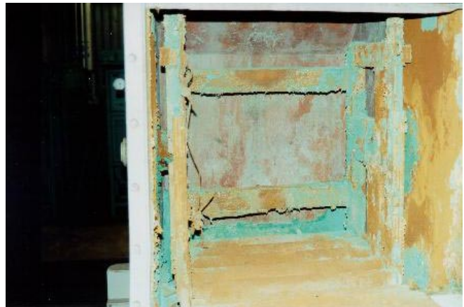
Quantities of uranium materials are clearly evident at product handling points in Building 340.
