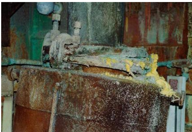
One ash receiver in Building 410 remains in place after 22 years, held in place by corroded C-Clamps. Uranium materials were clearly migrating from the receiver.
