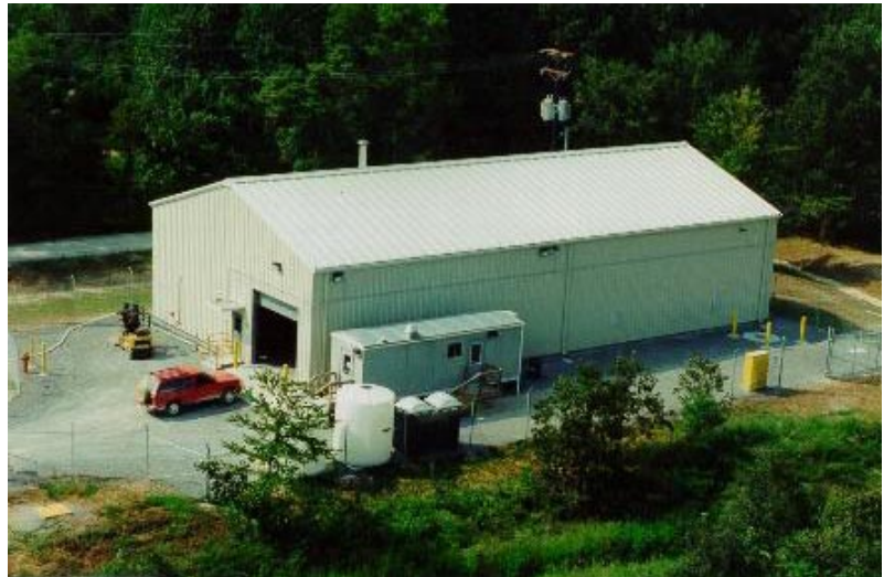
The pump-and-treat facility for the Northeast Plume was installed to slow the spread of TCE.
