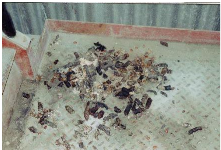
Animal material in Building 340 poses potential health effects to workers.
