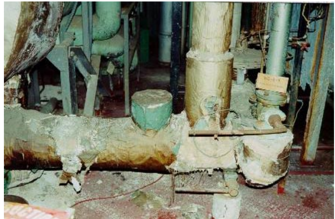
Many locations in shutdown buildings contain degraded lagging probably containing asbestos.
